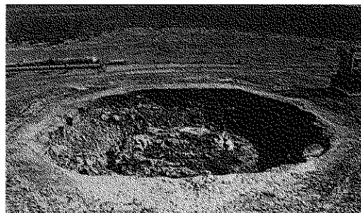
Photo 2 Depression Due to Volume Reduction (about 10m Diameter)
